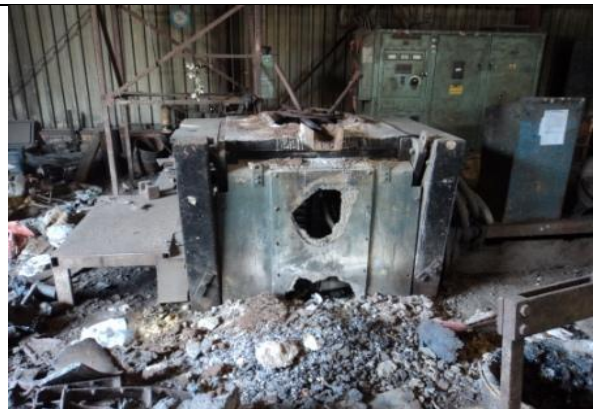
Fig. 4 Electric Furnace for melting Metals at Dhalaut Karyashala
